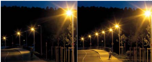
If one lamp is switched off or broken, the resulting dark area might be dangerous for the road users (especially pedestrians and cyclists).
